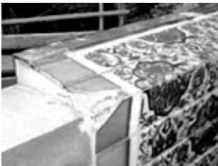
Broken blue border tiles prior to restoration. Note the face panel tile pattern continues onto the top level of the fountain. A thin copper water feed pipe will be installed across the top, flush with the edge of the blue border tiles. 06PWR Photo courtesy of Parker Jackson.
