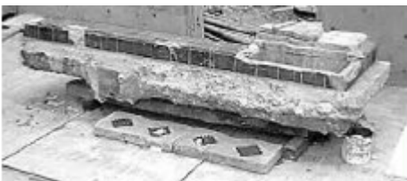
The original basin and recessed light well unit was moved back on site to insure accurate dimensions for the construction of the new basin. The original light well covers are seen in front of it. 07PWR Photo courtesy of Parker Jackson.
