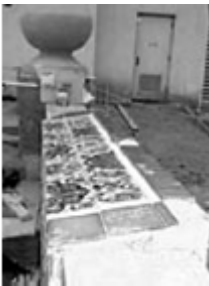
Missing blue border tiles (lower right and center), prior to restoration. 05PWR Photo courtesy of Parker Jackson.
