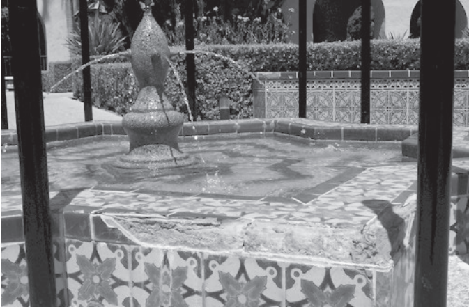
Damage to tile fountains in the Alcazar Garden
