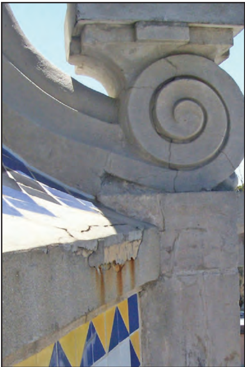
Typical cracks in stonework. Photo by Curtis Drake.
